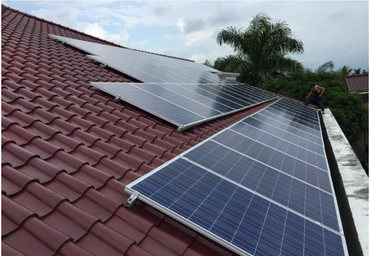
*Joya Residence, Pasig. – 11 kWp grid-tied installation
